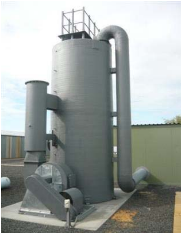
Dry Scrubber, Busselton, Australia
