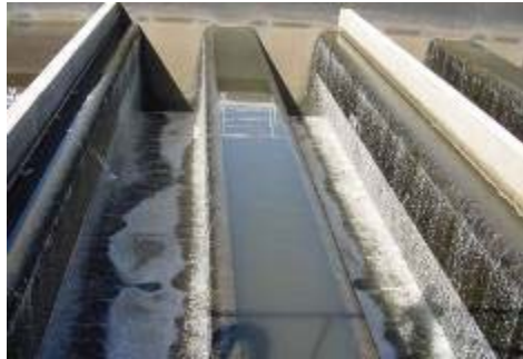
TETRA® Denite® Denitrification System
