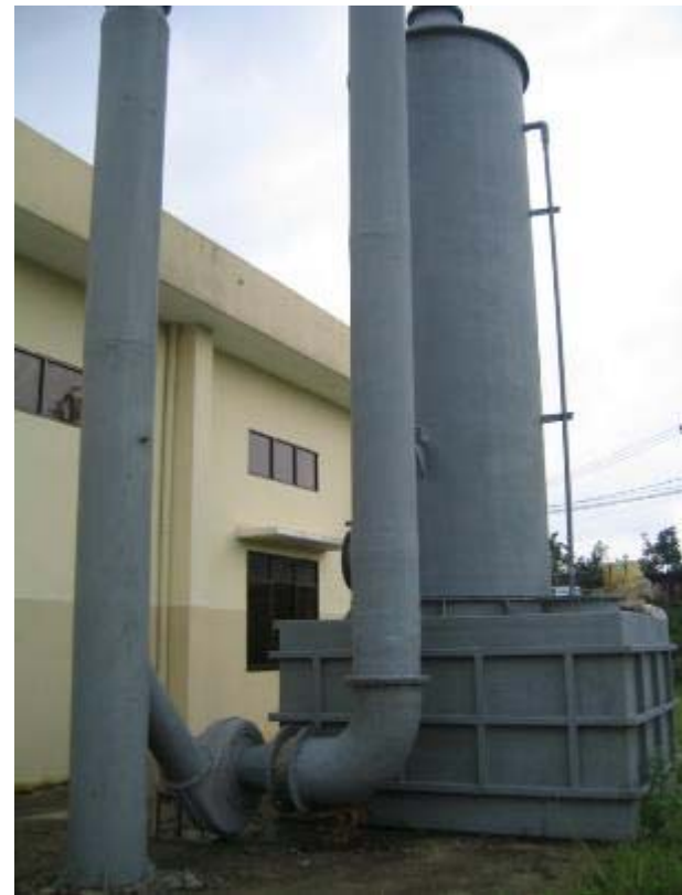
Wet packed tower scrubber, Cau Do, Vietnam
